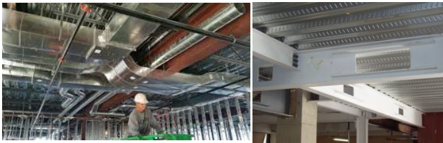
Figure 24: Services accommodations within false ceiling head room.
