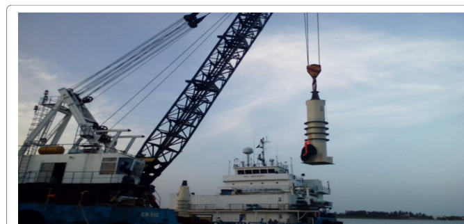
Figure 1: Works currently ongoing at Ada Foah (Source: TCs Energy Limited of Ghana).
