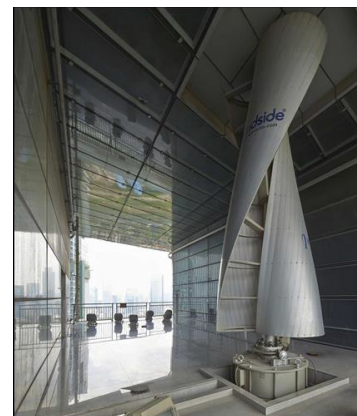
Figure 9: A turbine in one of the four intakes in the Pearl River Tower [24].
