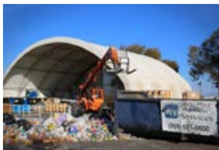
Figure 1: CleanWorld's anaerobic digester biorefinery which processes 40,000 tons of food waste annually for the production of biomethane for transportation applications.
